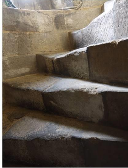
Example of uneven step
