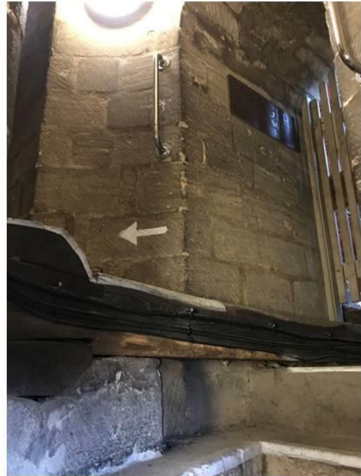
Trip Hazard: Beam. Step to the right, use handles to climb over
