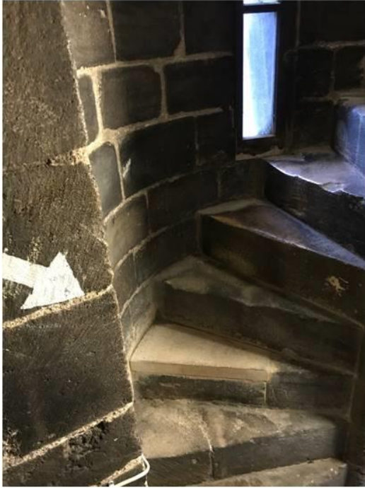
Staircase to tower is narrow and has no hand rail
